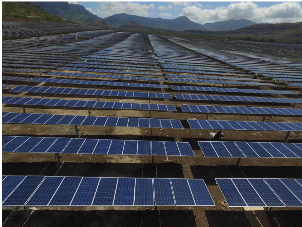
Figure H-4. Waianae Grid-Scale Solar Facility on O'ahu (close-up detail)
