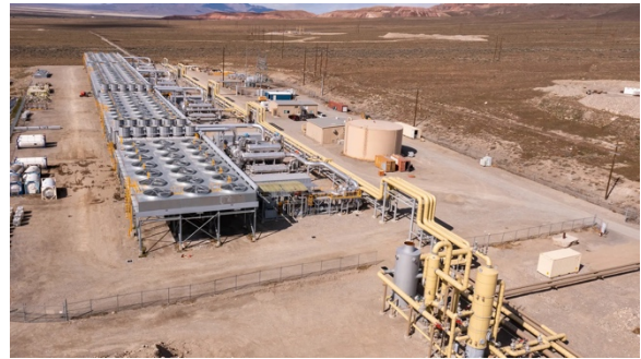
Figure 19. Star Peak Geothermal Energy Project
