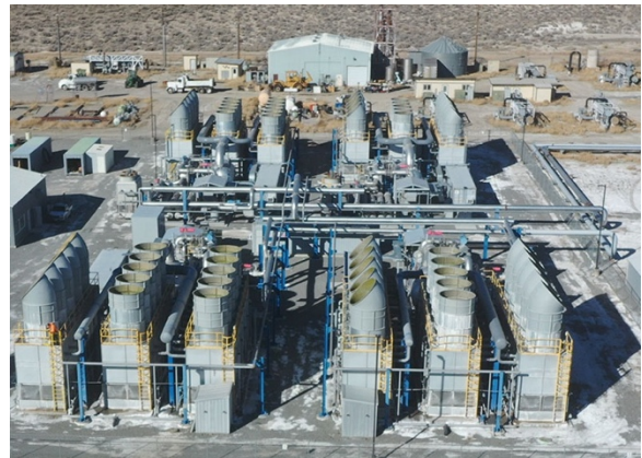
Figure 20. Whitegrass No.1 Geothermal Plant
