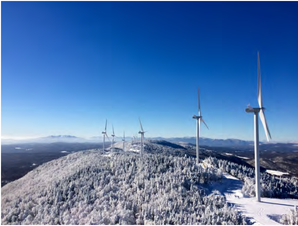
Figure 5-14. Granite Reliable Wind Facility
