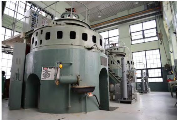
Figure 5-5. Fairfax Falls Hydro Turbine Generators
